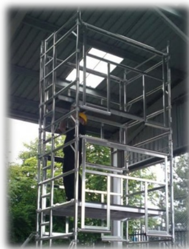
14. Remove the temporary trapdoor platform Position to the appropriate rung (Trapdoor facing the ladder section) 1 rung above the bottom section of the AGR frames.
