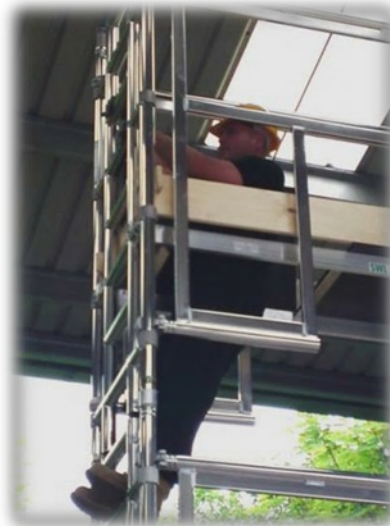
10. Access and egress to the next platform level through the trapdoor, using the ladder provided.
