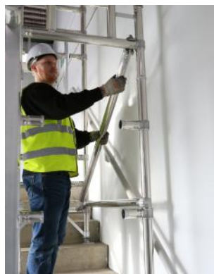
Fit another diagonal from the bottom rung of the ladder portal frame to the top rung of plain portal frame on the right hand side.
