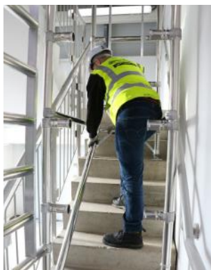
Fit diagonal brace from bottom rung of ladder portal frame to bottom rung of plain portal frame, on the left hand side.
