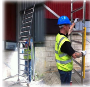
3. Add next set of frames and engage the interlock clips. Level the structure by adjusting the leg nuts as required.
