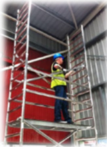
11. Fit 2 diagonal braces running in opposite directions starting from the rung in between the guardrail braces.
