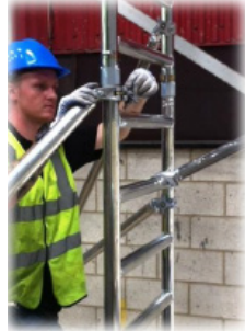
6. Secure stabilizers as low down as possible to increase tower stability, adjust according to the guide for larger towers or to overcome obstacles.
