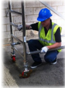
2. Fit 2 horizontal braces to the vertical member of the frame as low down as possible.
